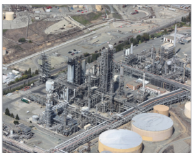
refineries and wellhead
